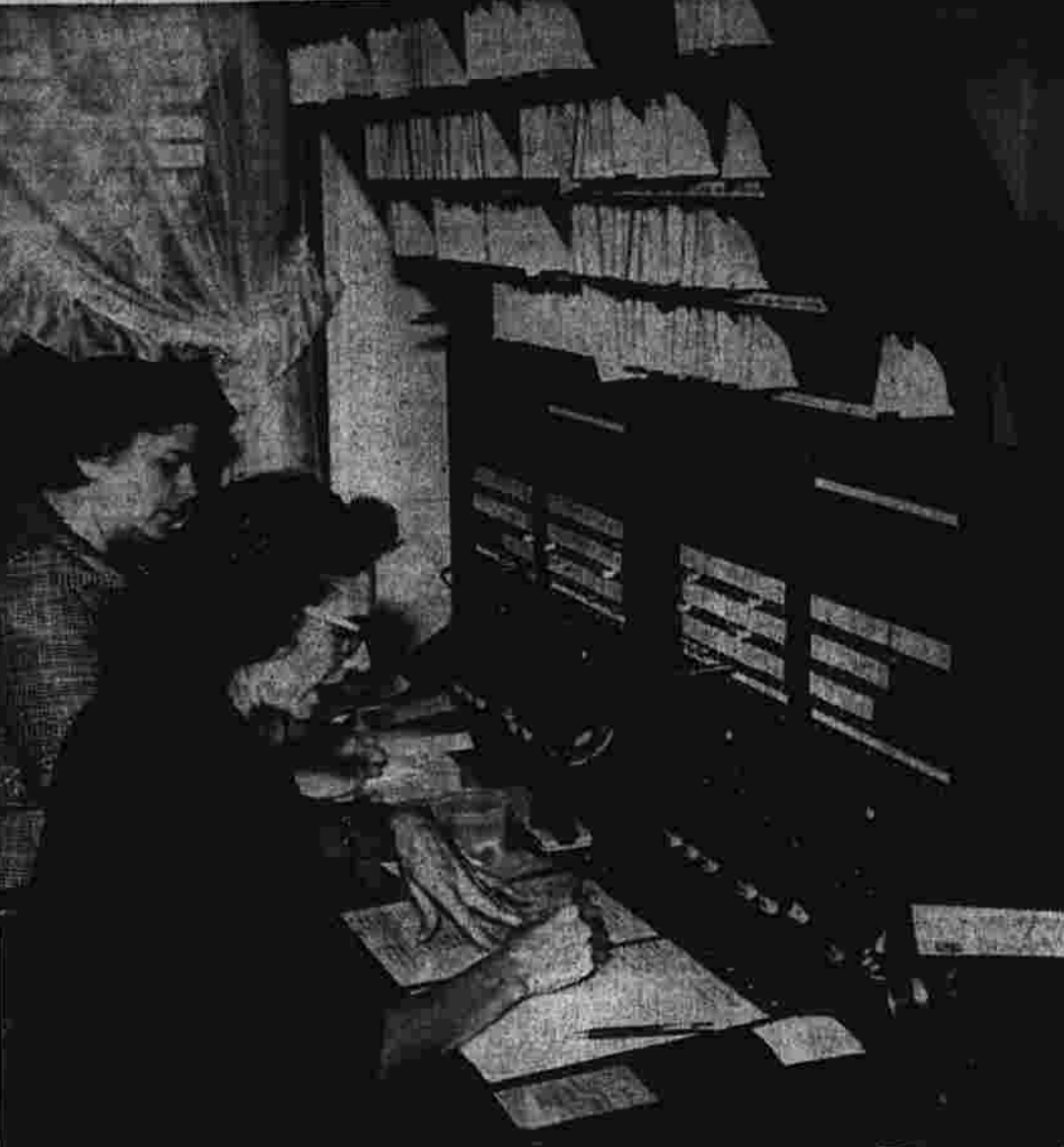
Mrs. Betty Ruth Edwards, rear, and Mrs. Annette Anderson of Taicottville, take calls on the new compact switchboard at the Manchester Answering Service, 318 E. Middle Tpke. The board has some 12,000 incoming and outgoing calls a month of which four to five thousand are recorded. (Herald photo by Saterlin).
